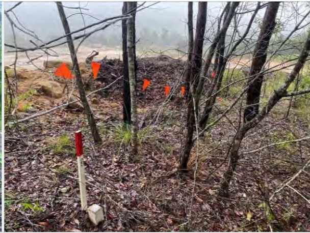
CLEARING PHASE IMAGE RETAINED HABITAT BEHIND VEGETATION PROTECTION FENCING AND MULCH BERM.
