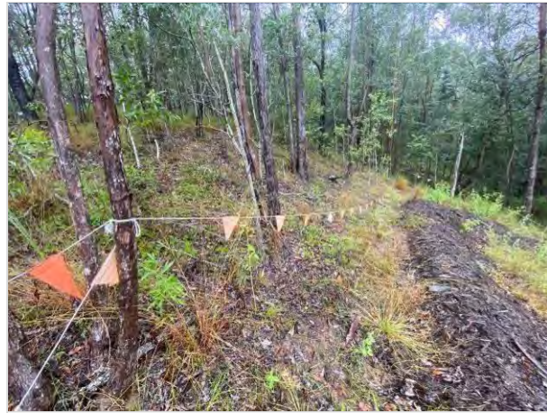
CLEARING PHASE IMAGE RETAINED HABITAT BEHIND VEGETATION PROTECTION FENCING AND MULCH BERM
