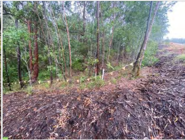
CLEARING PHASE IMAGE RETAINED HABITAT BEHIND VEGETATION PROTECTION FENCING AND MULCH BERM.
