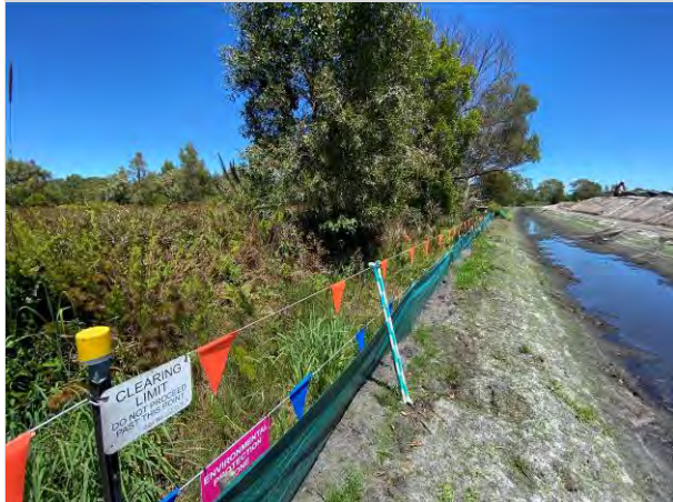
Vegetation Protection Fencing, Signage and Silt Fencing Installed at the Interface Between Retained Frog Habitat Zone and Construction Area
